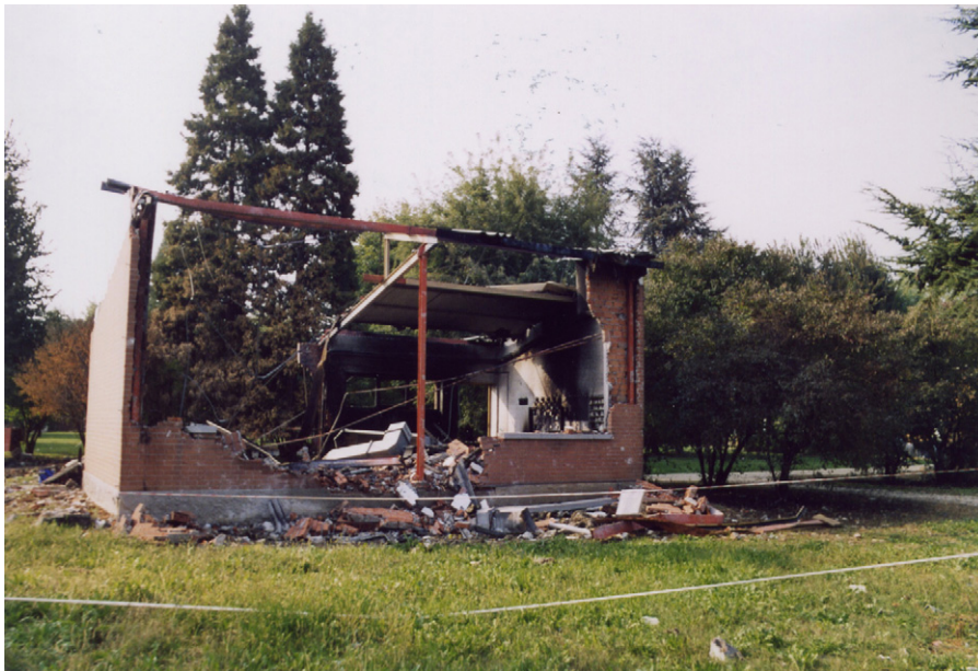
Photograph 4. Damages in the surroundings.
